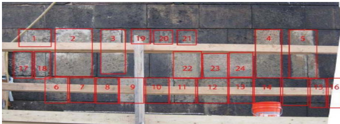
Testing samples at the High Bridge . Photo courtesy of JMC Stone Co.
